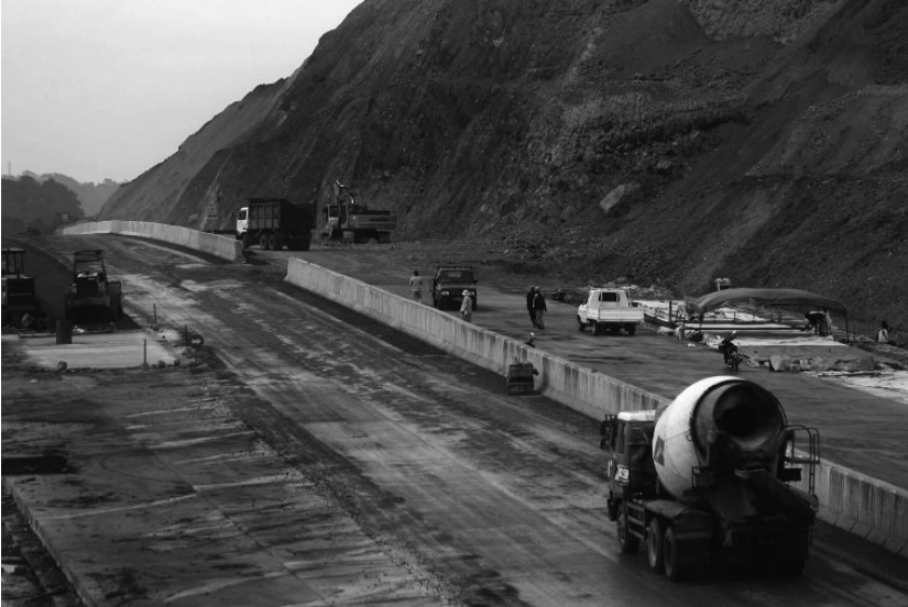
Figure 6.3 Taming the hilly, rugged terrain of the Semarang–Ungaran section of the Semarang–Solo toll road in February 2011 ( Tempo /Budi Purwanto).
